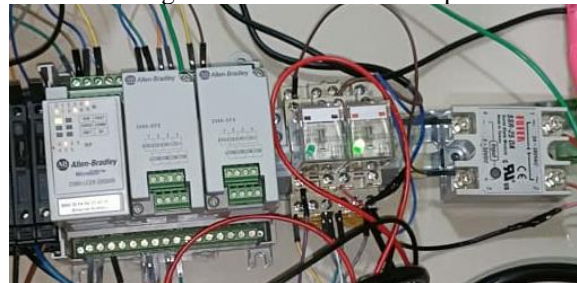
Figure 4. Control Panel Setup
