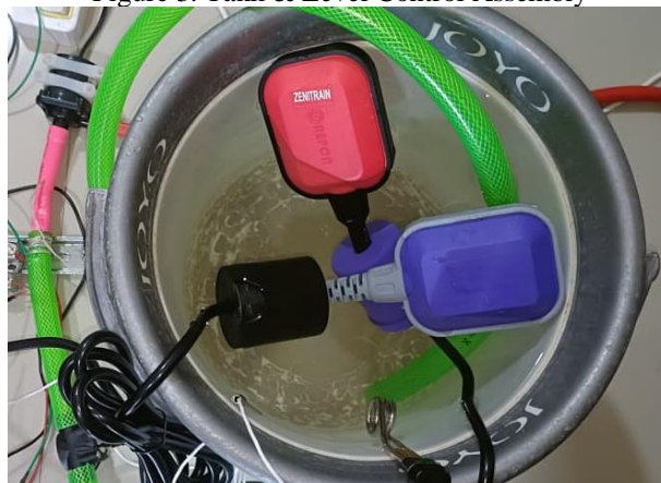
Figure 3. Tank &amp; Level Control Assembly
