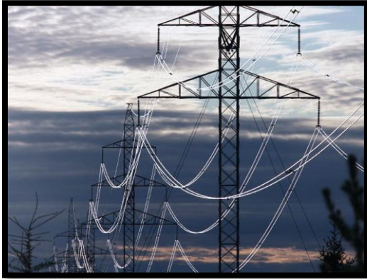
HVDC Power Line
