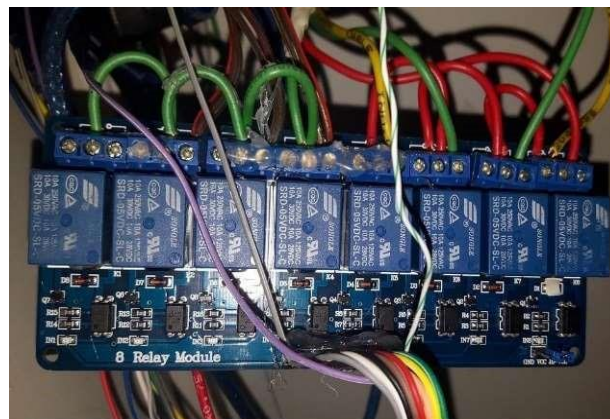
Figure .2 Relay board used in the proposed case (consists of 8 independent relays)
