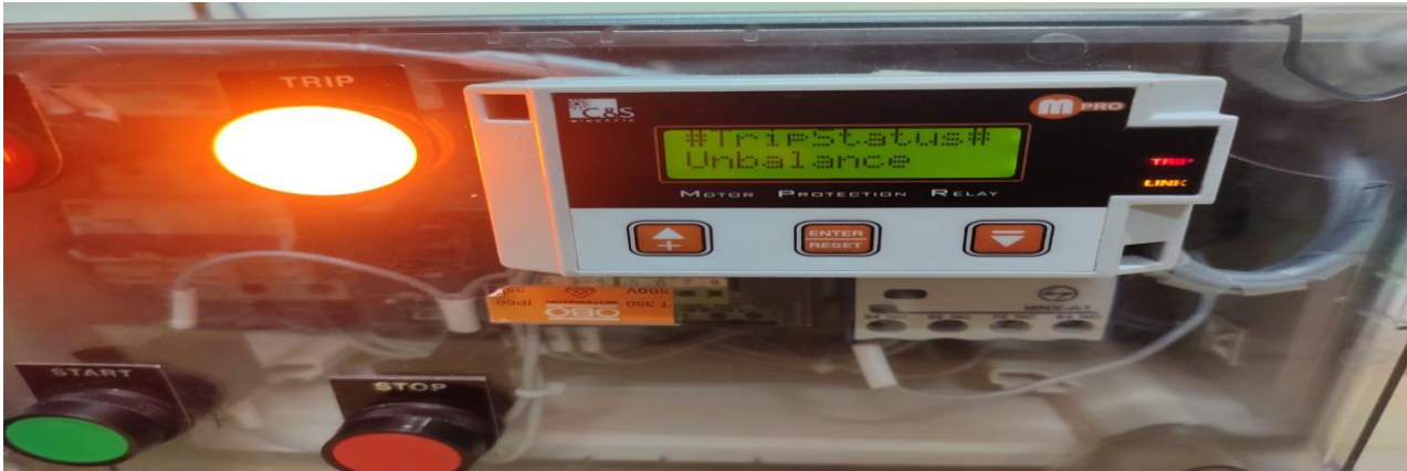
Fig.9 Unbalance tripping status
