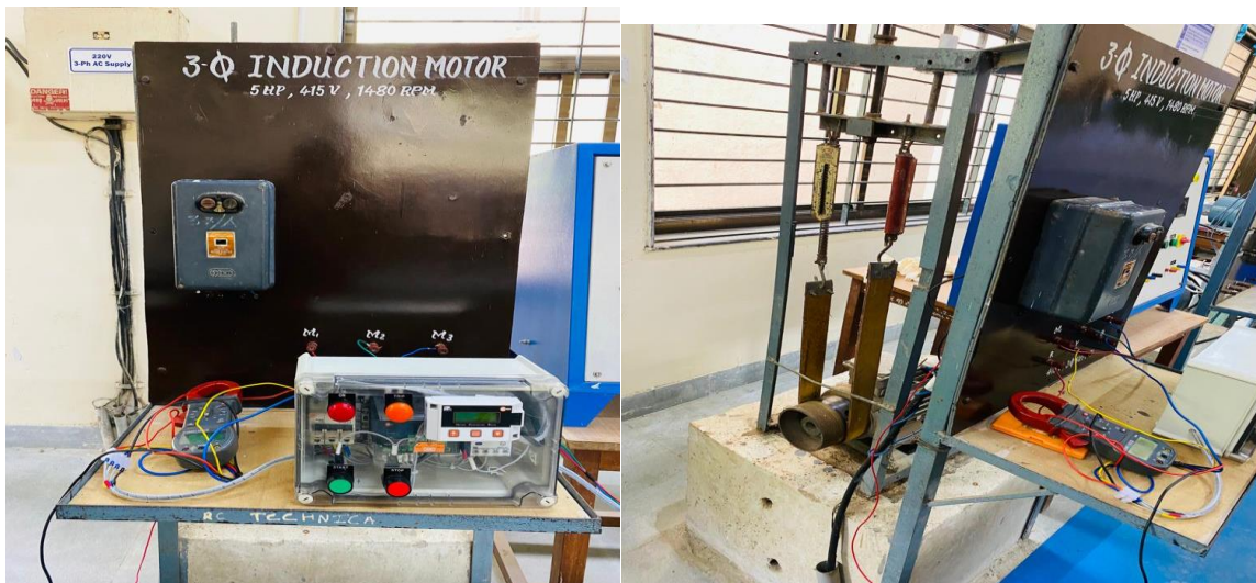
Fig.10 Testing of protection panel using Numerical relay on three phase induction motor
