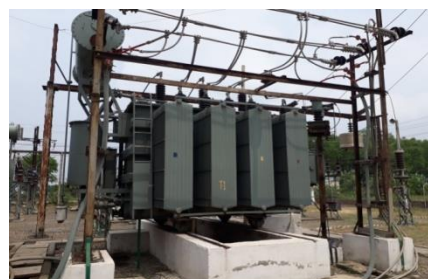
Fig.1 12.5 MVA Power Transformer
