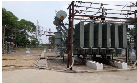
Fig. 2 10 MVA Power Transformer
