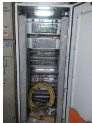
Fig 1. Remote Terminal Unit (RTU)
