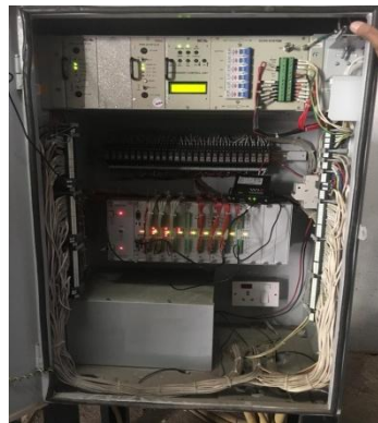
Fig 3. Feeder Remote Terminal Unit (FRTU)
