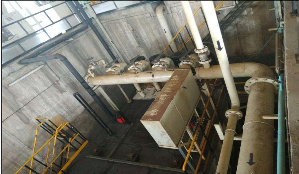
Fig.1: Coolant Filtration Plant
