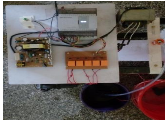
Fig. 7 Top View of Designed Prototype Model of PLC Based Car Wash System
