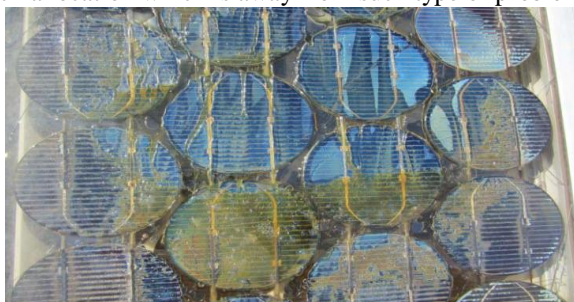
Fig. 7: Degradation of PV module
