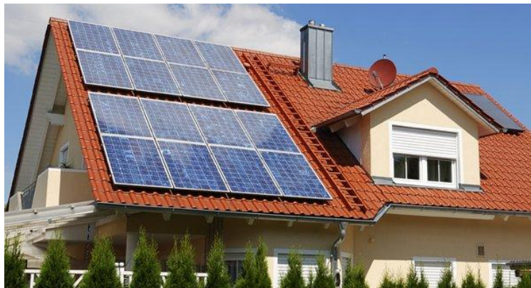
Fig.2: House rooftop Solar Panel
