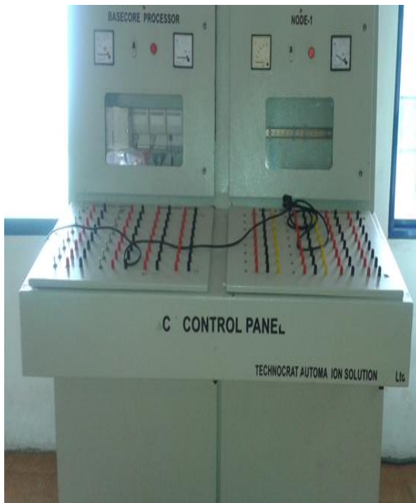
Fig 1 Local Control Unit (LCU)
