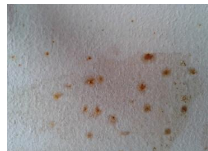
Figure1. Steel coating image with rust defects (Scene image)
