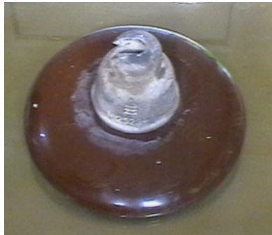
Fig. 1: A photograph of the porcelain insulator has been in service since 1986.
